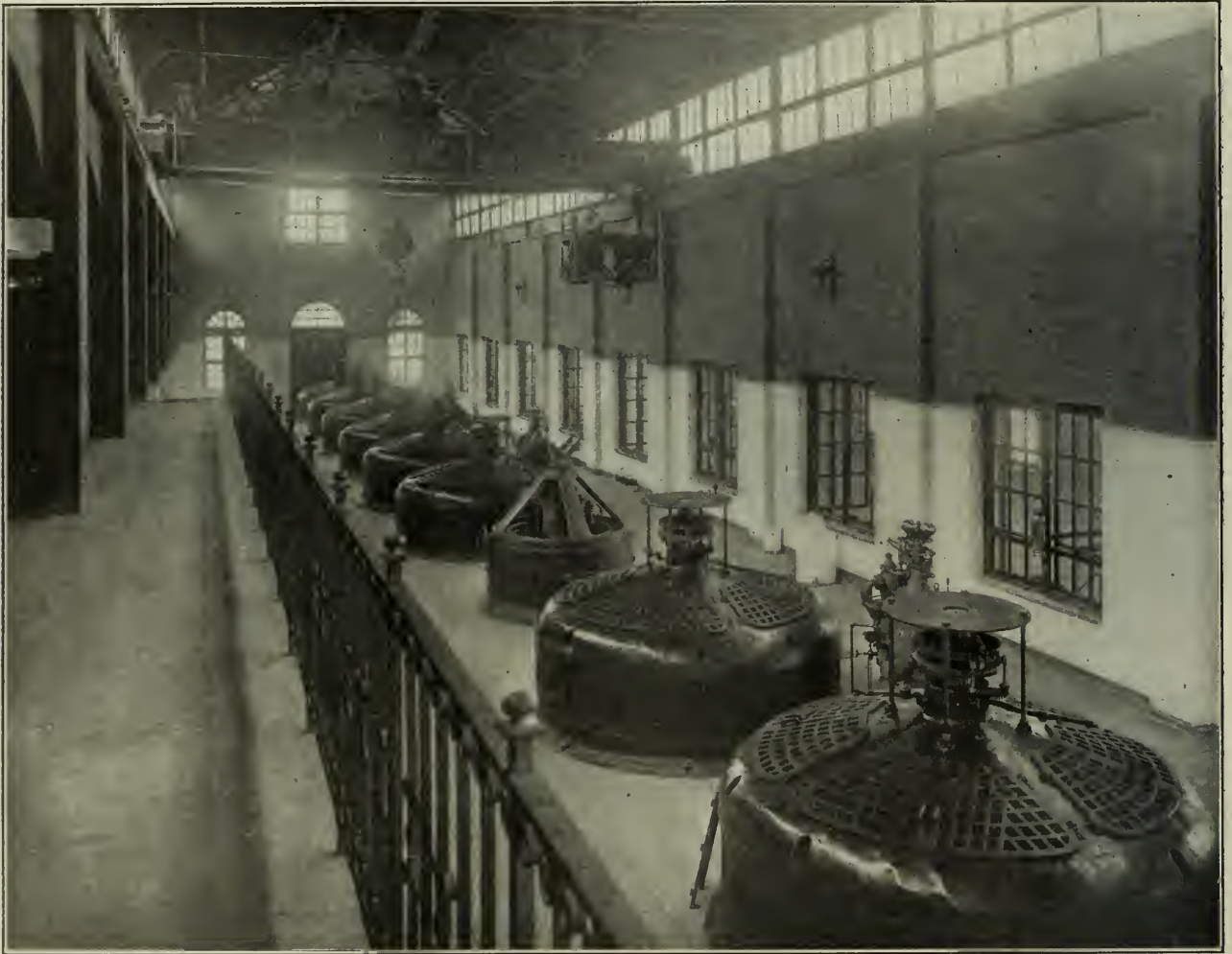
FIG. 3. THE GENERATORS AND EXCITER UNIT
